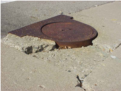
METAL OR OTHER PLATES, COVERS, OR GRATINGS THAT ARE NOT FLUSH (3/4 INCH OR MORE VERTICAL DIFFERENCE) WITH THE ADJOINING SIDEWALK SURFACE, ARE STRUCTURALLY UNSAFE, OR CAUSE A NUISANCE DUE TO SLIPPERY SURFACES ETC.
