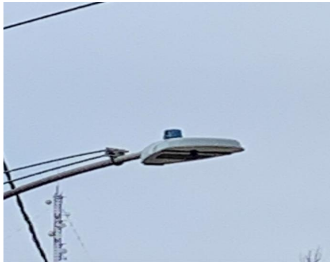
New typical LED light head – Miami Valley Lighting
